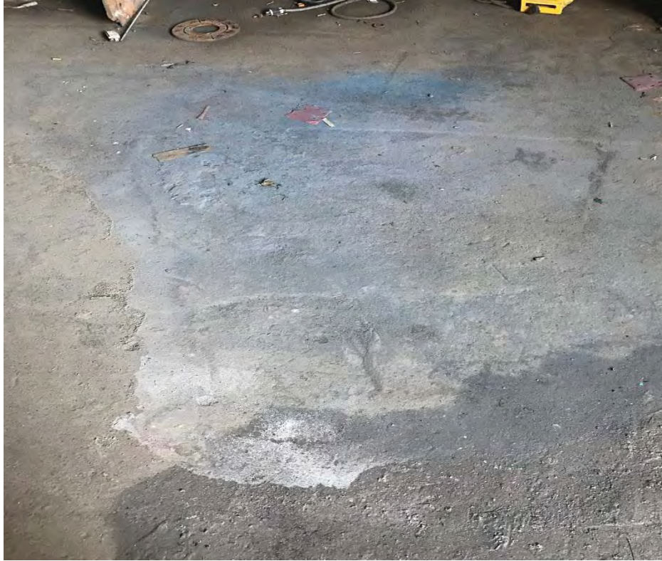
Figure 7: Paint staining inside the workshop.
