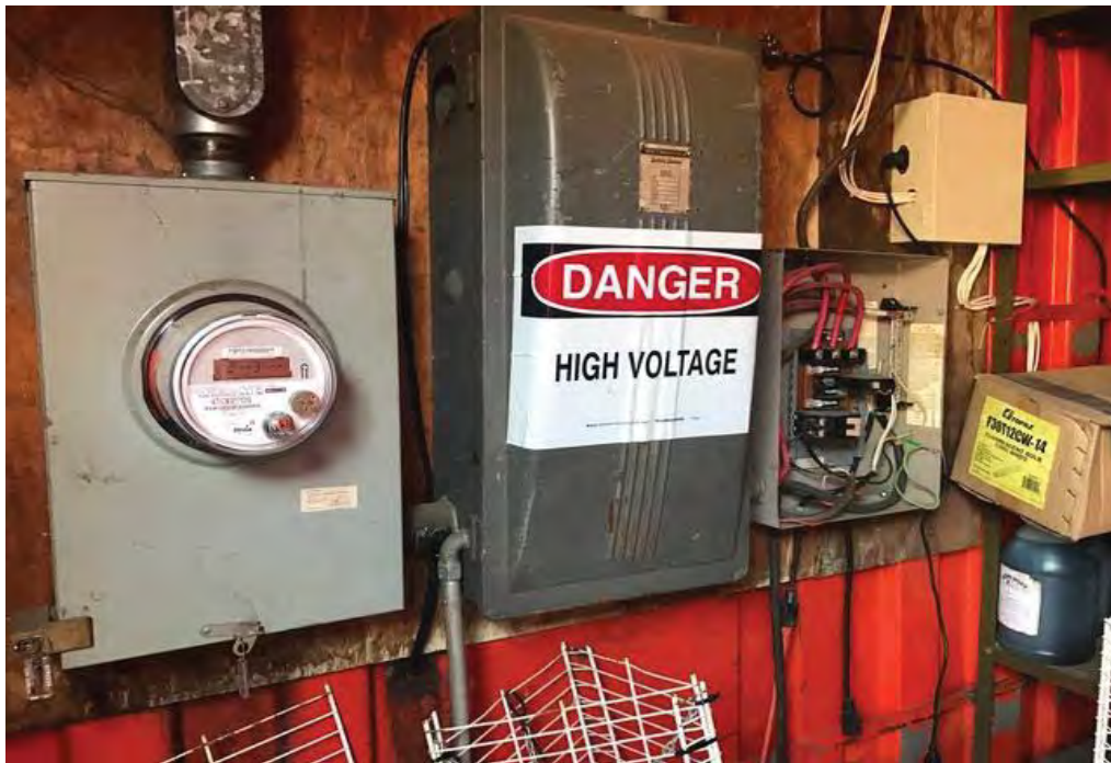
Figure 6: Electrical panels in workshop.
