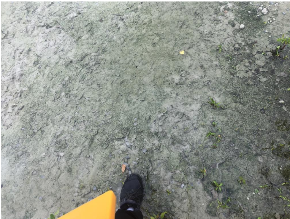
Photograph 8: View of concrete washout on the Subject Property.
