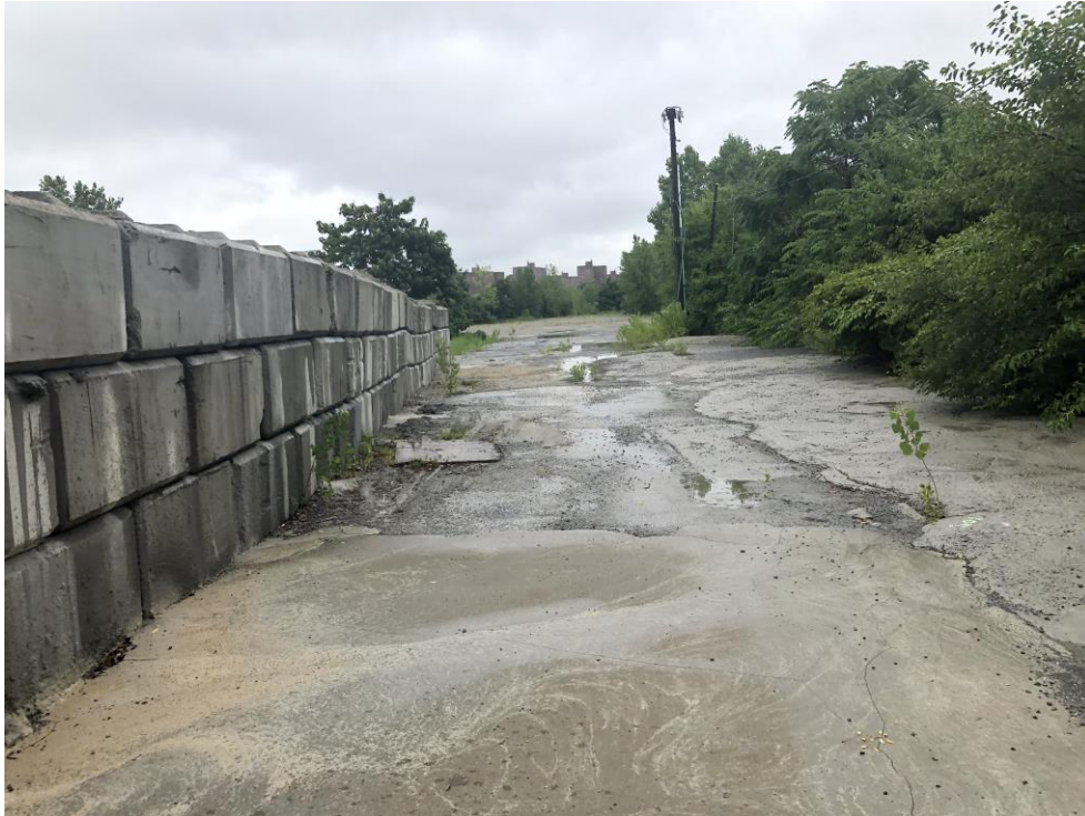
Photograph 7: View of unevenly poured concrete mix and stacked concrete blocks on Subject Property; facing northeast.
