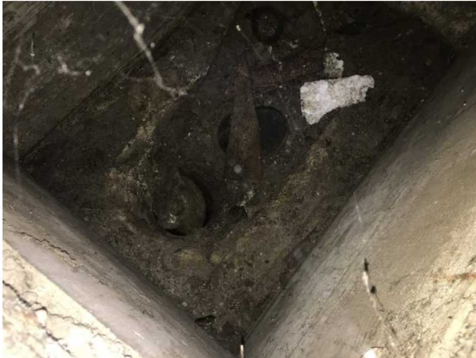
Photo 11: View of the tank inside the concrete vault beneath the entrance off East 144 th Street
