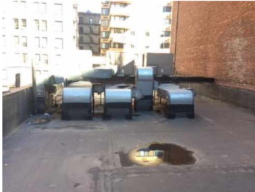
Photograph 9: View of the heating, ventilation, and air conditioning (HVAC) equipment on the roof of the Lot 59 building, facing north.
