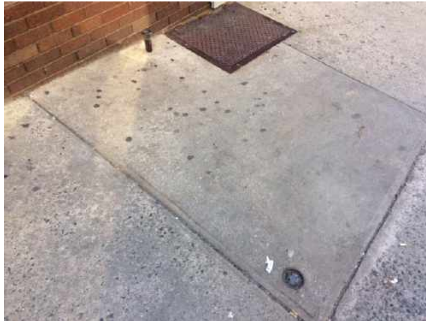
Photograph 11: View of the fuel oil fill port and vent pipe located on the sidewalk adjacent to the Lot 60 building, facing southwest.
