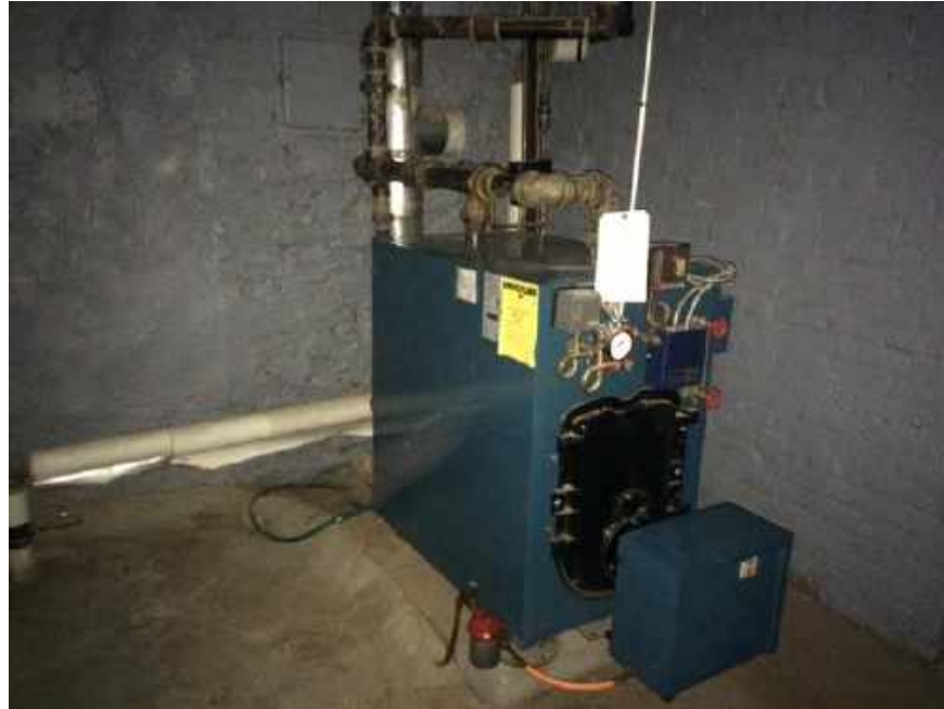
Photograph 13: View of the boiler room in the cellar of the Lot 60 building, facing east.
