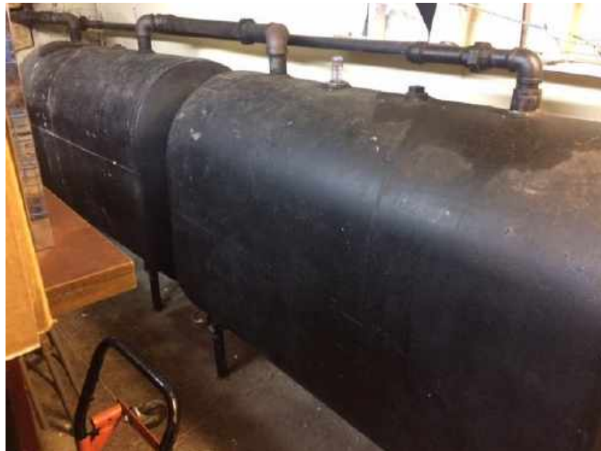
Photograph 14: View of the active 275-gallon aboveground storage tanks (ASTs) located in the cellar of the Lot 60 building, facing north.
