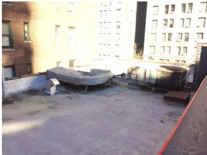
Photograph 18: View of HVAC equipment on the roof of the Lot 59 building, facing northwest.
