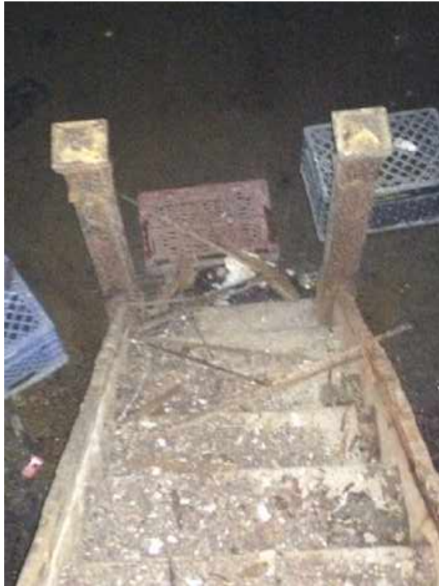
Photograph 3: View of the stairwell into the cellar level of the Lot 57 building, facing east.
